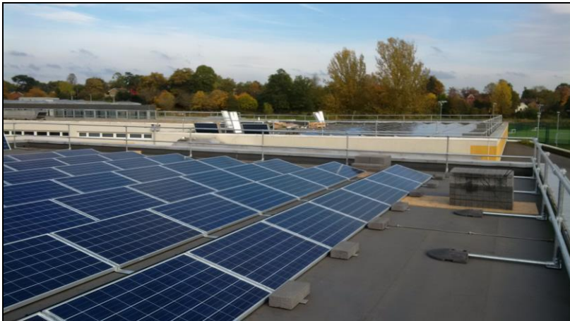
Garth Hill College using the Council Invest to Save scheme installed a 50 kWe Solar Photovoltaic system on the Sports Hall roof.
